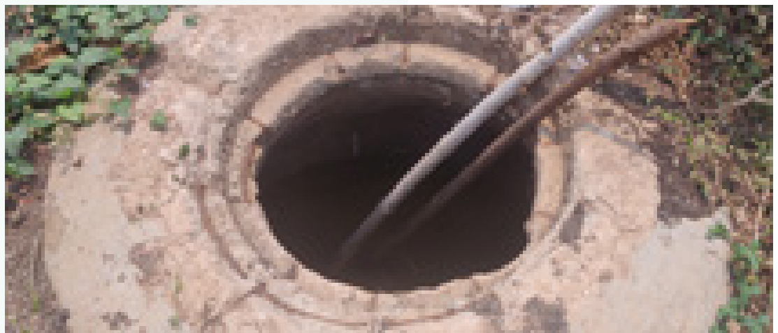
Figure 3: Desludging vehicle unloading Faecal sludge in a manhole
