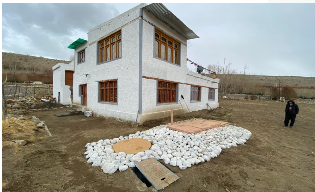
Figure 10: The greywater treatment unit
